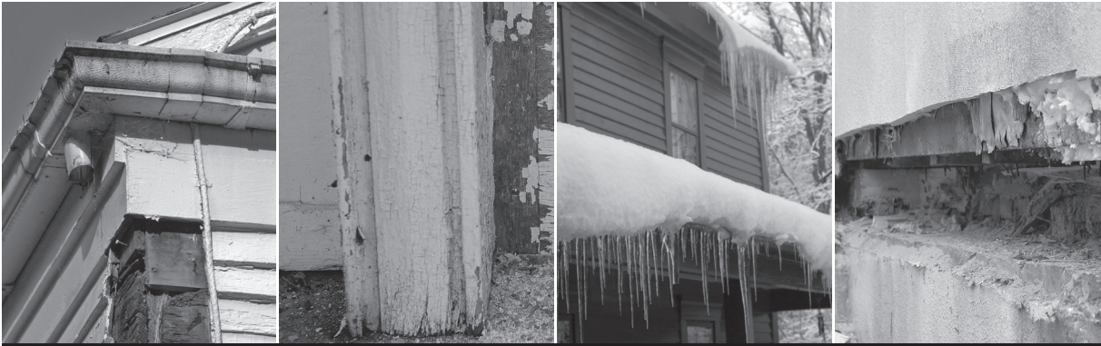
LEFT TO RIGHT: A clogged gutter and absent downspout drove water into this corner of the building, making it necessary to replace the post at a cost of thousands of dollars; water splash off the granite threshold has rotted door trim work; ice dams caused by heat leaking out of a building can drive water under building materials; moisture penetration has left this sill rotted.
