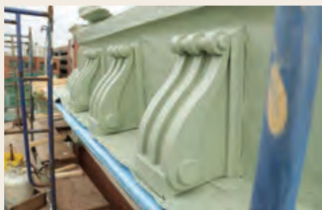
Copper cornices have been restored as part of the comprehensive rehabilitation of the former Grand Trunk office, also a federal tax credit project.
