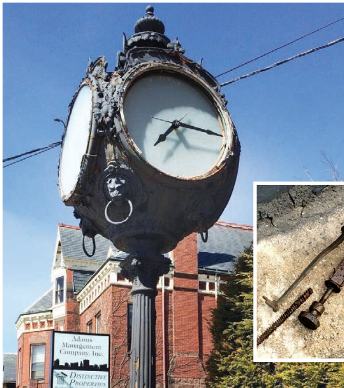
The early 20th century Seth Thomas street clock on Congress Street stopped working decades ago due to a lack of maintenance and exposure to Maine's harsh environment.
