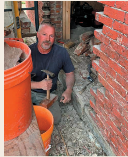
A member of Richard Irons' masonry crew works on the brick restoration.
