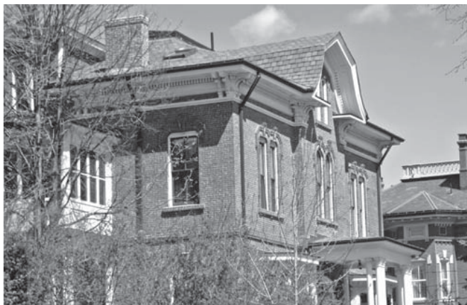
A slate roof like this one poses many challenges, with its multiple angles, gutters, flashing, decorative trim, and skylight. Repairs are often best left to a qualified professional.
