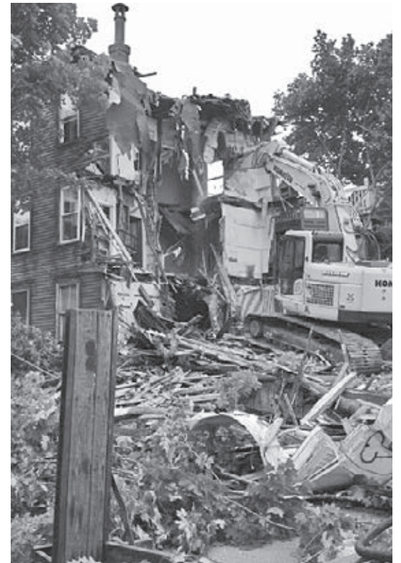
Demolition of this property on Newbury Street took place in June, highlighting the vulnerability of India Street's historic fabric.
