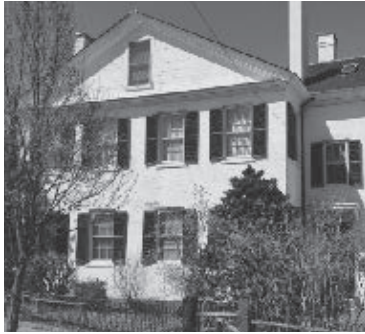
Shrubs close to a building can trap moisture and cause mildew and rot.
