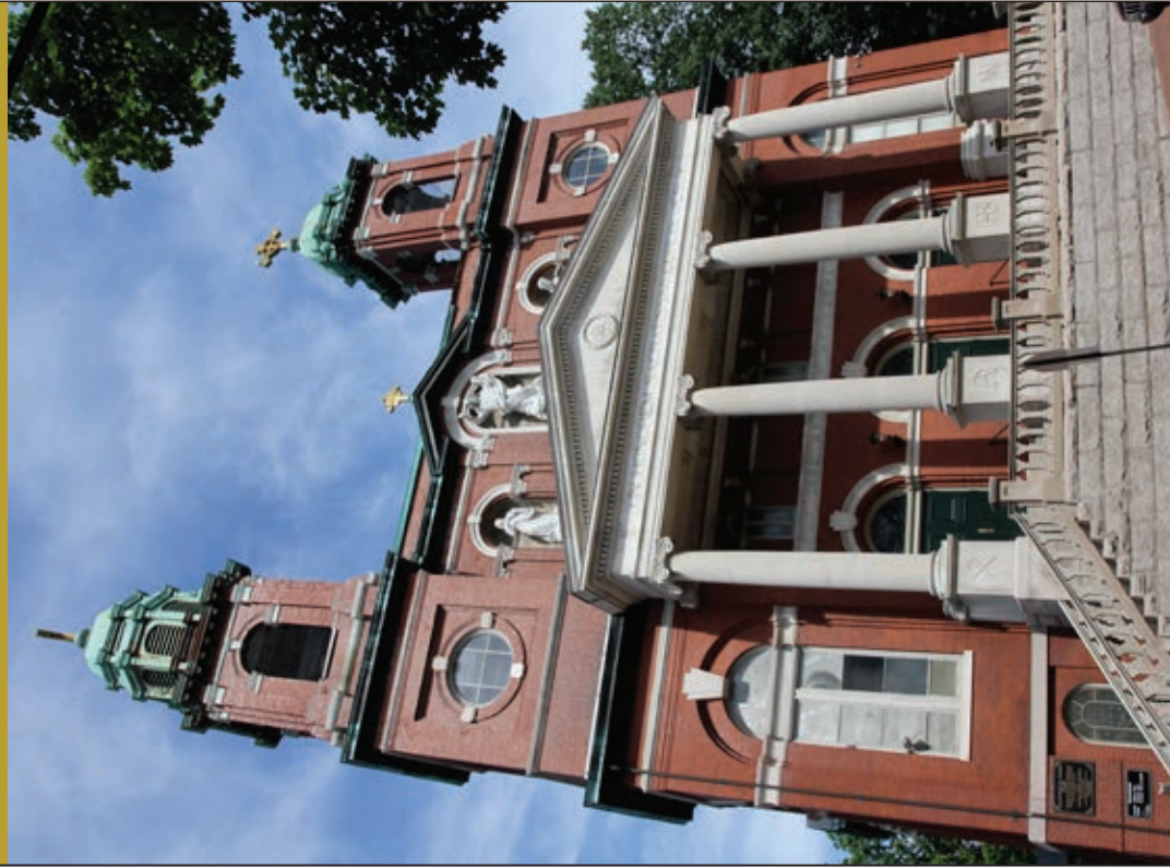
The Church of the Sacred Heart (1886-1915) on Mellen Street in Portland, designed by Francis Fasset, is one of five local endangered properties cited by Landmarks in 2015. An active congregation is raising funds to repair the leaking copper roof on the apse to preservation standards.
