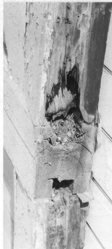
Figure 5. Some internal core deterioration was masked by sound surface wood. Water entering the connection of the post and beam framing rotted out the mortise and tenon pockets. These areas were consolidated and filled with epoxy. Photo: Baird Smith, AIA
