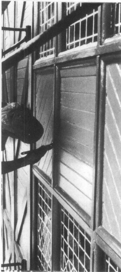
Figure 9. The building was painted with two coats of oil-alkyd primer and two top coats of acrylic latex. Photo: Bryan Blundell
