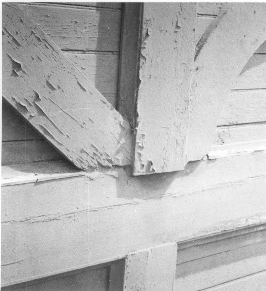
Figure 4. Flaking paint was the result of painting moisture-laden wood, using an inappropriate paint system, and undertaking the work during cold weather. Photo: Baird Smith, AIA
