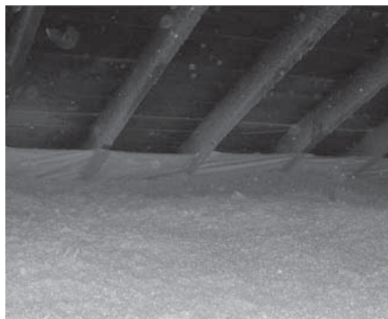
Attic insulation can be a preservation strategy to avoid ice dams and reduce energy consumption.
